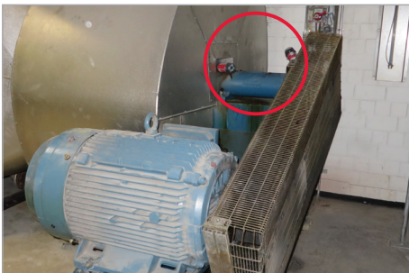
Lubrication of bearing unit on a fan
