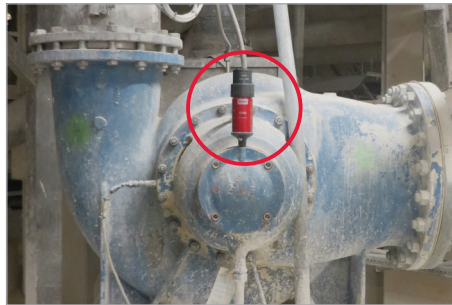
Bearing lubrication on a pump
